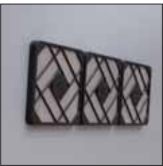
Inlet and exhaust fans with filters
